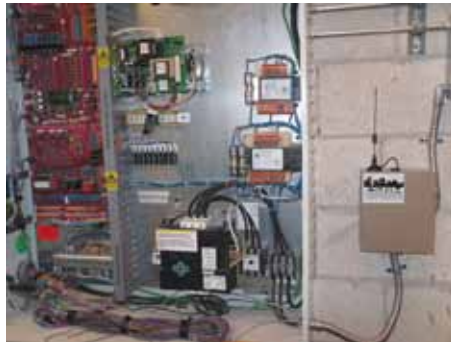
An Elevator Connect 1000 (right) mounted in a machine room
