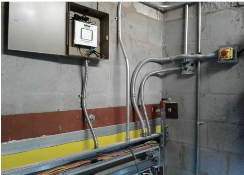
The EC1000 enables emergency phone service through a cellular connection without the cost of extra infrastructure.
